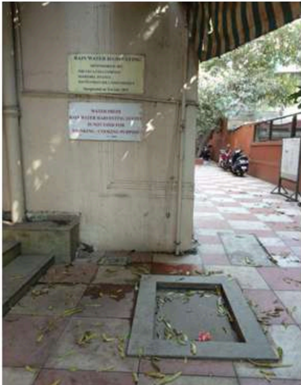
Rain Water Harvesting
