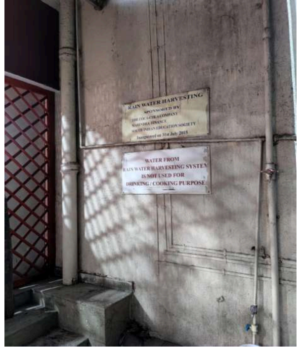
Rain Water Harvesting
